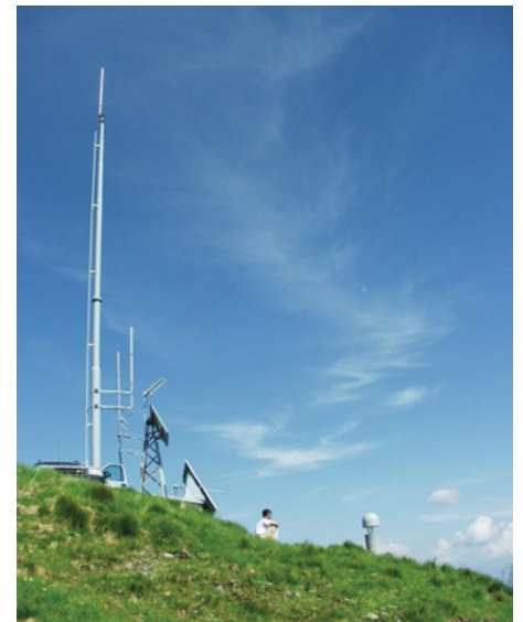
Fig. 2. GPS site installation at Zouf Plan (ZOUF) is shown. The station is located on a Carboniferous dolomite outcrop. The typical network monument (shown on the right side) consists of a 1-m concrete pier attached to surface bedrock using epoxied metal rods. The choking antenna is attached to the monument using an antenna adapter and is covered by a dome. The antenna cable is trenched to a nearby structure housing the seismic data loggers and GPS receiver. Cellular modems are used to telemeter the data once per day, using the SHARC/EGADS data acquisition software to control the data retrieval.
