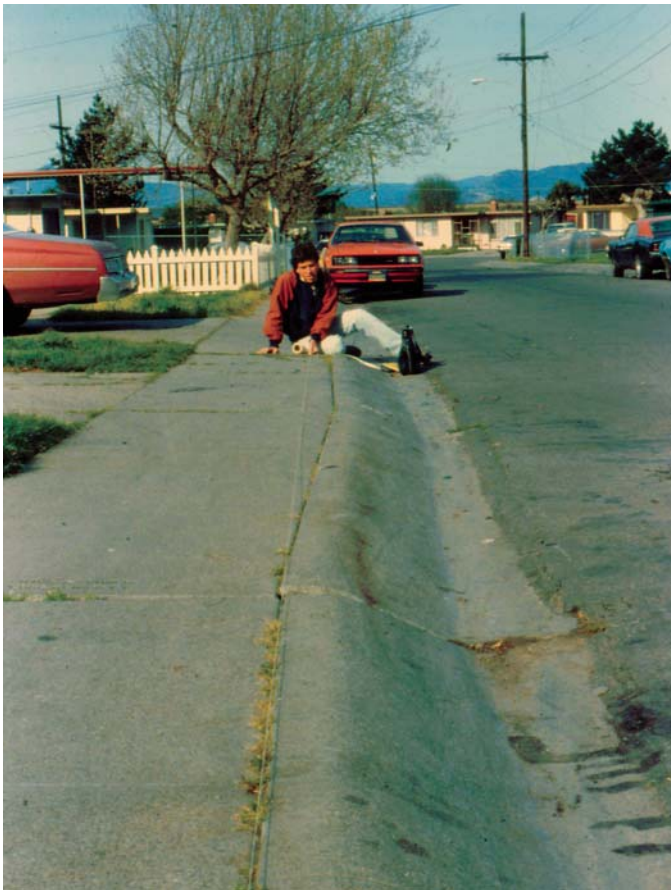
Figure 24. Right-lateral curb offset at 704 Phanor Drive due to aseismic slip in Parchester Village that was 150 mm (6 inches) by 21 March 1985. More precise techniques found 214 mm of offset in a wider span of the northwestern curb on Banks Drive in 1988 (Lienkaemper et al., 1991). By now, the offset should be about twice as much as shown here. Gene Kelley, Colorado State University, for scale.
